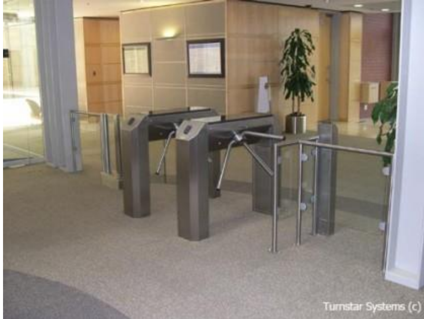
Figure i: Typical installation with barriers and screen
